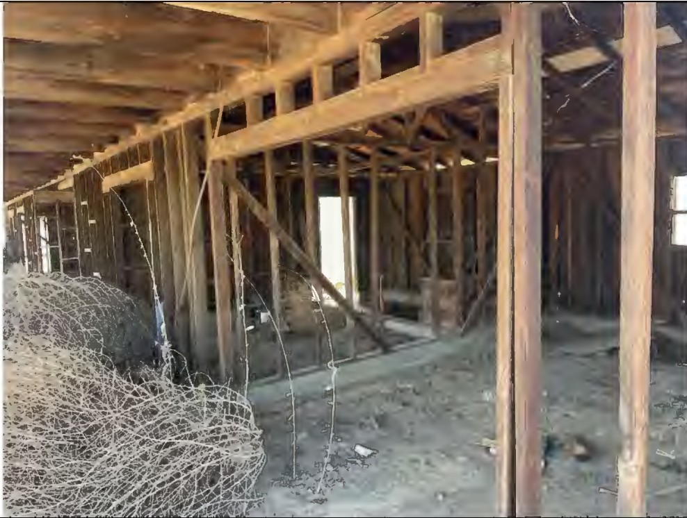
Photo #5 Interior view of stables in the central portion of Subject Property.
