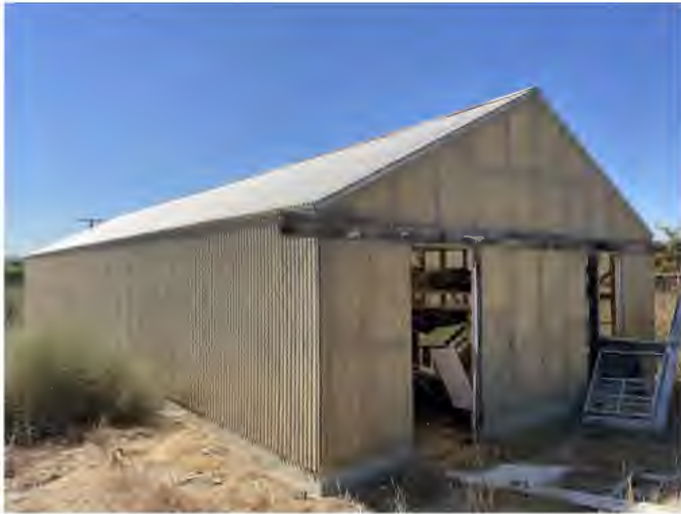
Photo #7 View of vacant greenhouse in the northwestern portion of the Subject Property.
