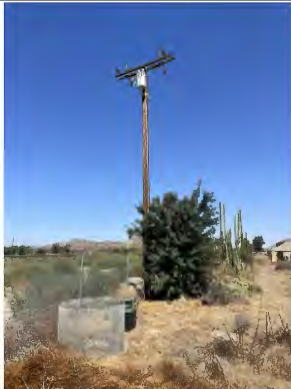
Photo #6 View of pole mounted transformer in the northwestern portion of the Subject Property.
