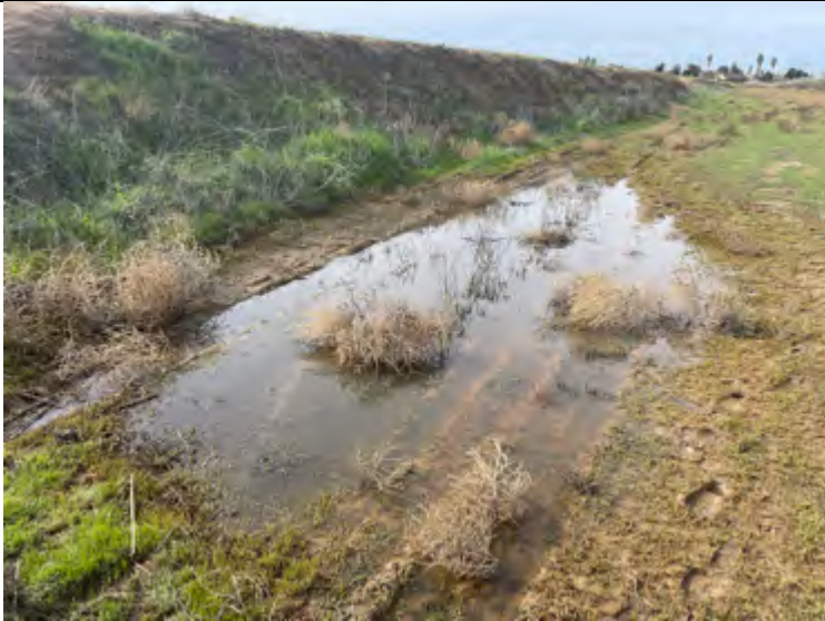
Photograph 2. View of Basin 8 in northwestern portion of project area (taken 1/13/23; facing west).
