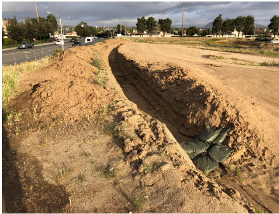
Figure 8: Photo of Drainage Channel Running East to West on Southwestern Corner of Project.
